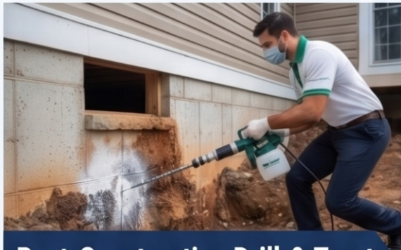
Post-Construction Drill & Treat
